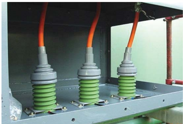
Installed Capacitive Couplers
