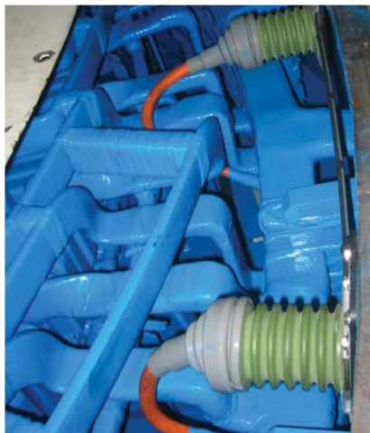
Couplers installed on a hydro generator stator
