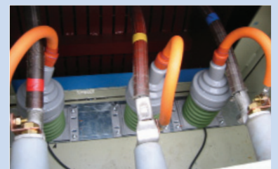
Installed 80pF PD Couplers
